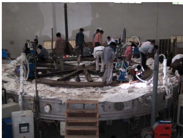
Fig. 19: The bottom plate of PFBR Grid Plate mounted on the preheating furnace with hardfacing in progress
